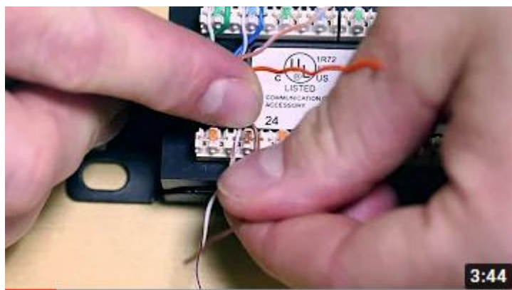
Figure 21 - Video about mounting a copper patch panel
